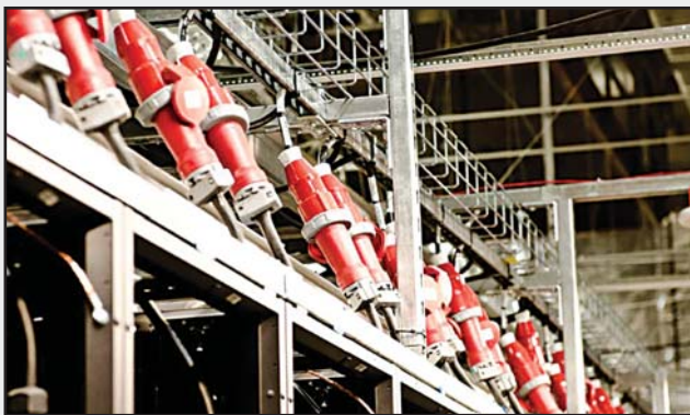
The Intergate.Columbia data center, Wenatchee, WA, BlackRock build out. The racks are populated with dual 415/240-Vac plugs.
