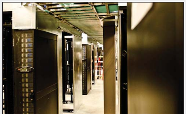
The Intergate.Columbia data center, Wenatchee, WA, BlackRock build out. Shown here are 415/240-Vac modular IT power distribution units.
