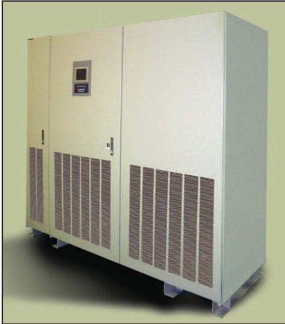
Online double-conversion UPS system downstream of a standby generator with complete electrical isolation between the power source and the critical load
